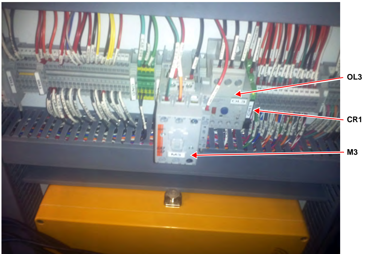
Figure 14: Driller's Cabin Wrench PLC cabinet
