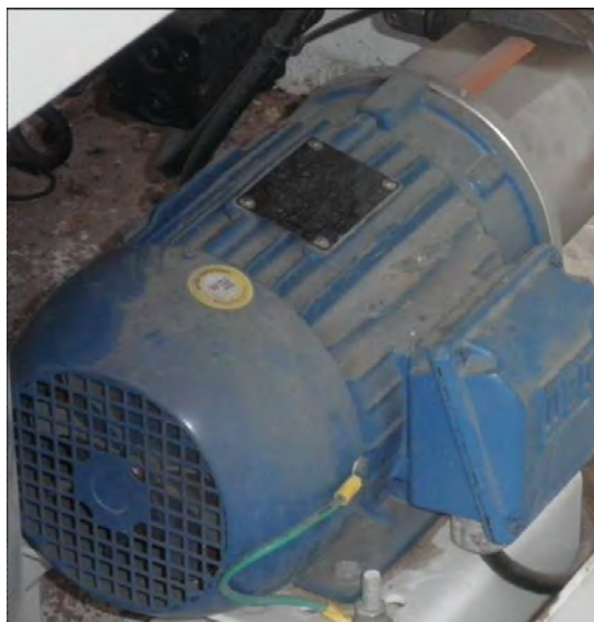
Figure 2: Blue- Weg # 00218ET3E145TC, three phase motor.
