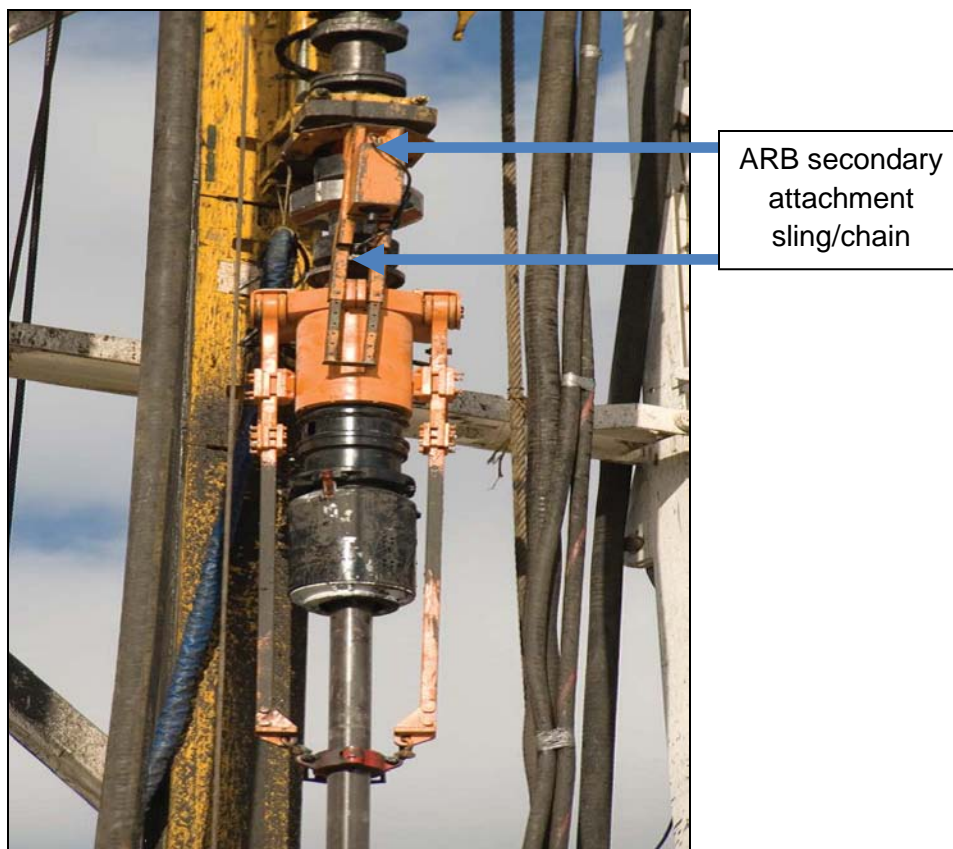
Figure 1: An ARB may fall onto the rig floor if it is not properly attached with a secondary fail safe such as a chain or sling
