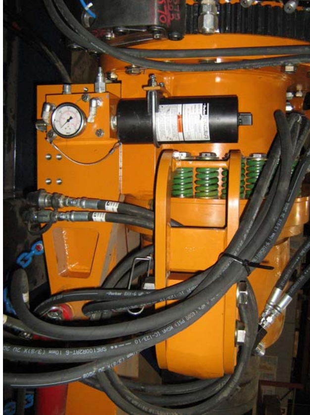
Figure 2 – Relocated Accumulator, Clamp Bracket and Safety Cable
