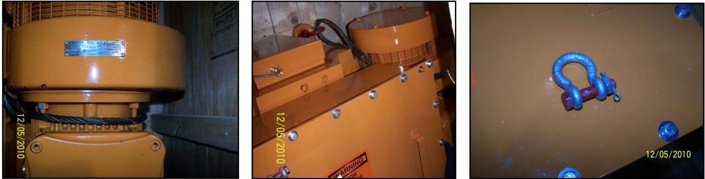
Figure 4: Securing the blower motor assembly using a wire rope sling as a secondary retention
