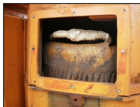
Figure 3: Sheared mounting bolts on 600HP induction motor air intake
