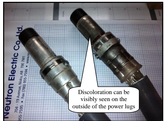
Figure 3: Discoloration on the outside of the power lugs
