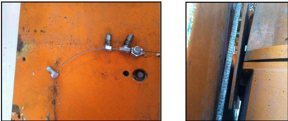
Figure 2: Bolts that have come loose or failed, causing the motor junction box to slip on the TESCO EXI-600 Top Drive
