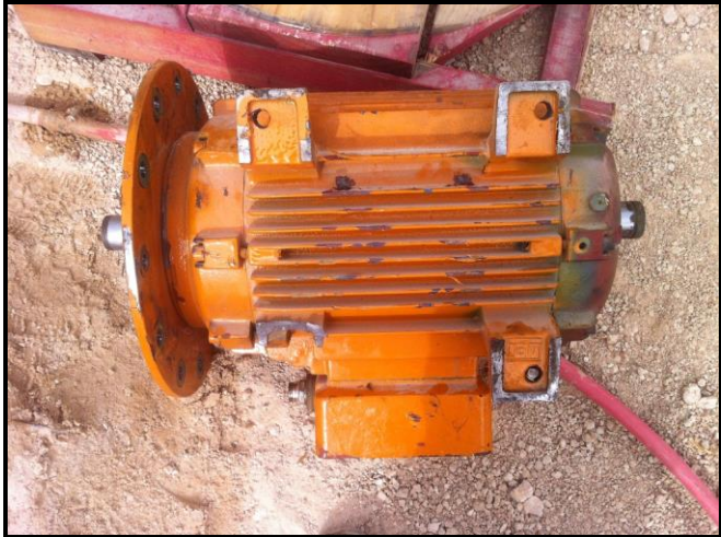
Figure 2: Mounting foot of blower motor failed
